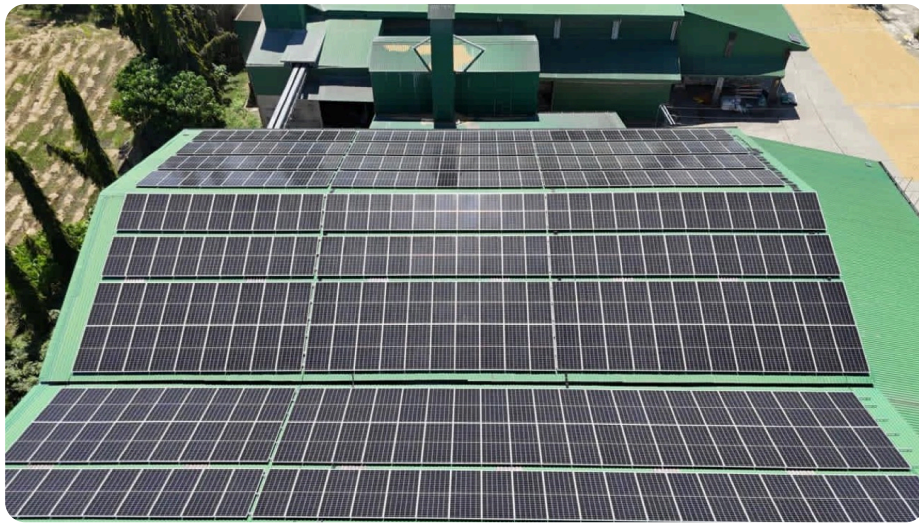
ON-GRID ARRAY CARRYING THE DAYTIME INDUSTRIAL LOAD AT THE VM AGBAYANI RICEMILL.
