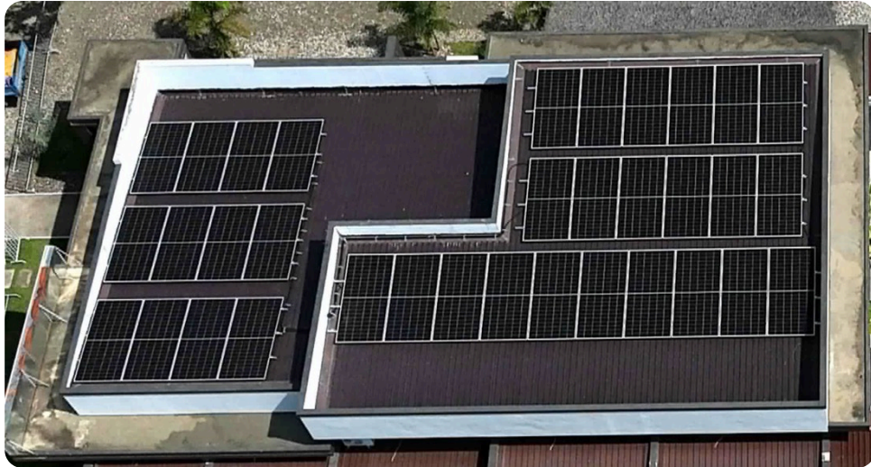
ROUND-THE-CLOCK RESILIENCE: HYBRID SOLAR AND BATTERY STORAGE AT DR. FONTE MEDICAL CLINIC AND PHARMACY.
